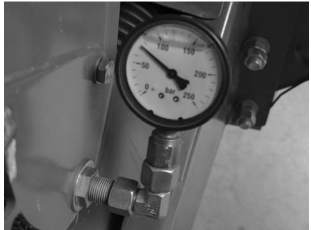
Figure 9.14: Pressure gage at cable guide via towing bar
